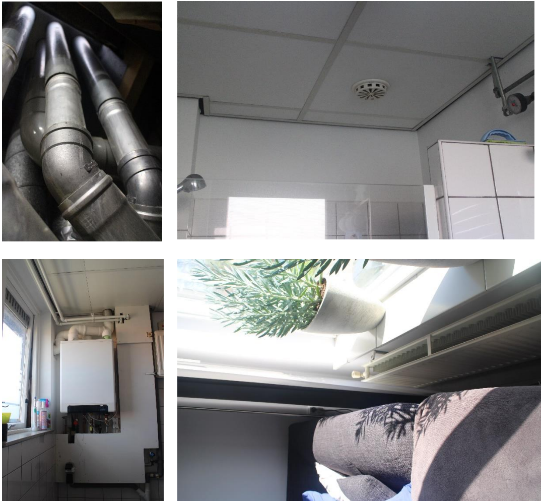
Figure 4.1.5: Building services exhaust: pipes, gas boiler and radiator, Source: Climate-KIC, 2017.
