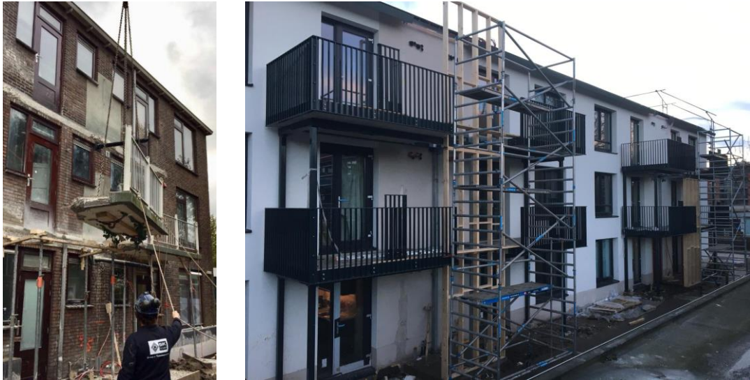
Figure 5.3.6: Removal of old balconies and the placement of the new ones, Source: Climate KIC, 2017.
