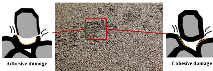
Figure 1.2 Ravelling failure modes.
