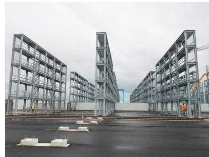
Figure A-4: Reefer racks at APM Terminals Rotterdam
