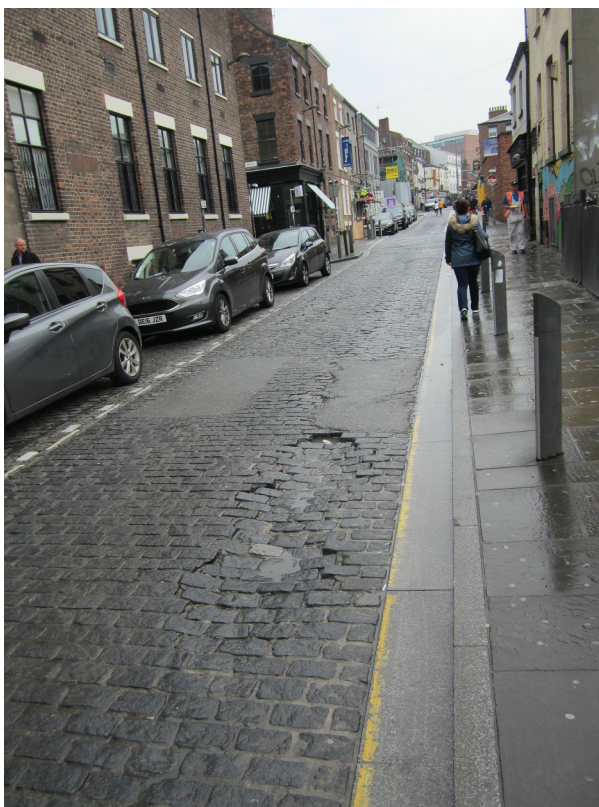
Figure 6. Cobbled street in poor condition in the Ropewalks. Photo by authors.
