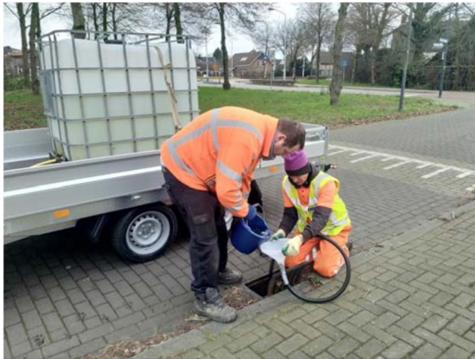
Figure 6.17 Pouring cold water onto the cable, in the underground sewer, using a hose and a funnel for validation of the measured distances by the DTS system. Source: courtesy Remy Schilperoord (Partners4UrbanWater).
