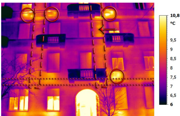
Figure 7 - Detail of the temperature distribution on the area around and above the main entrance (Case Study 2). The thermogram shows the heat loss due to the different thickness of the masonry, its finishing, and the location of heater/pipes.
