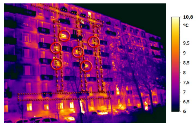
Figure 5 – Thermogram of the eastern façade of Case Study 2; outdoor air temperature 8 C, emissivity 0.92.
