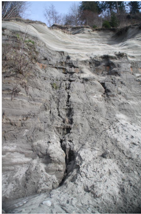
Figure 2.2: Gully formation in Point Grey cliff due to surface water run-off. Photo courtesy of S. G. Pearson.
