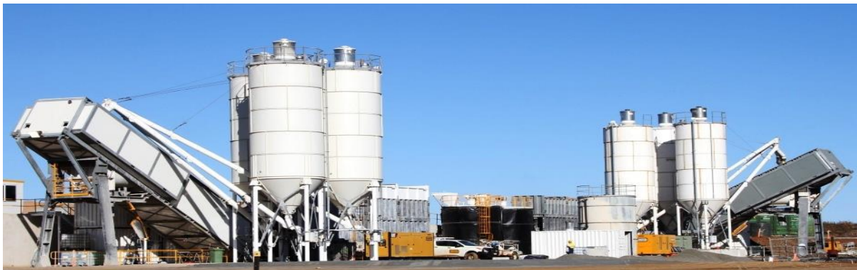
c) BWWA: twin mix batch plant
