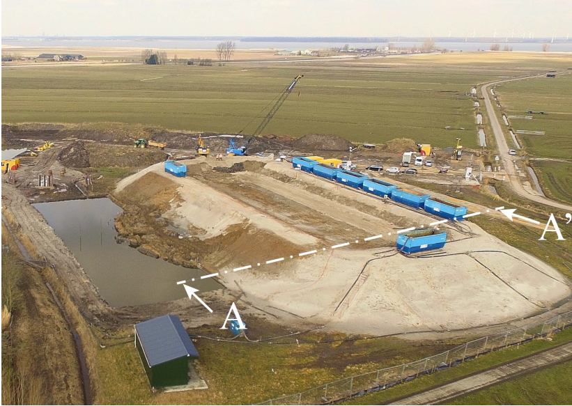
Figure 4.7: Aerial photo of the Eemdijk ring-shaped test dike, with slope instability of the conventional (ground) dike (left). The test dike with sheet pile, is located on the right side. Photo courtesy of Eric Feijten / NOS (Feijten , Photographer)
