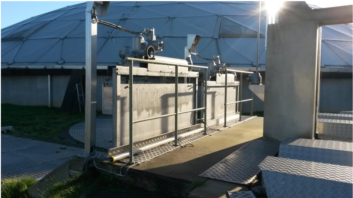
Fig B.2. Picture of the controllable valves to dynamically operate the PCs in the Primary Clarifier Control
