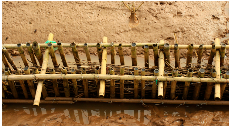
Figure 1. Wooden fences in the field [6]. The construction includes the frame (two rows of 6–8 cm diameter bamboo poles) and the inner part (a bunch of branches of 1–2 cm diameter bamboo reeds). Reproduced with permission from Dao et al. (2018), Journal of Coastal Research ; published by BioOne, 2018.
