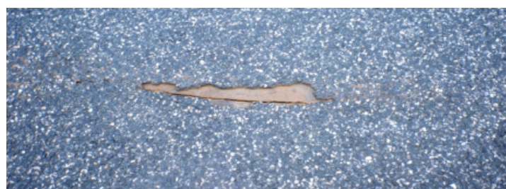
Figure 2.9: Deck plate crack on the Van Brieneoord bridge. The crack initiated at the weld root of the deck-to-trough joint and propagated through and along the deck. Its length is approximately 50cm [10]
