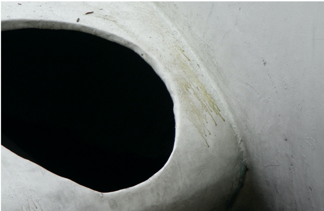
Figure 18. Leaching next to the joints by Maropol (Photo by Piero Medici, 2011).
