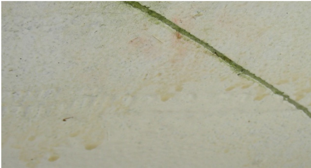
Figure 24. Close-up of the drops next to a surface opening (Photo by Piero Medici, 2011).
