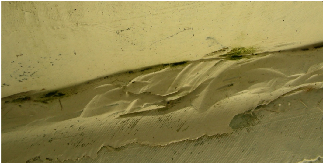
Figure 6. Close-up of finishes with epoxy resin, glass fibres and white paint coating. In the right part of this picture the spot is visible where the piece of Figure 5 was removed (Photo by Piero Medici, 2011).
