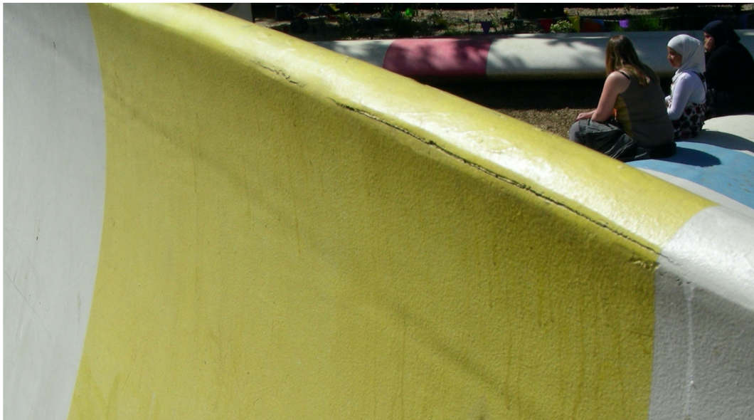
Figure 16. Leaching on the surface facing south-east of the blade standing on the long side. Drops seemingly coming out from an opening of the coating by Maropol (Photo by Piero Medici, 2011).
