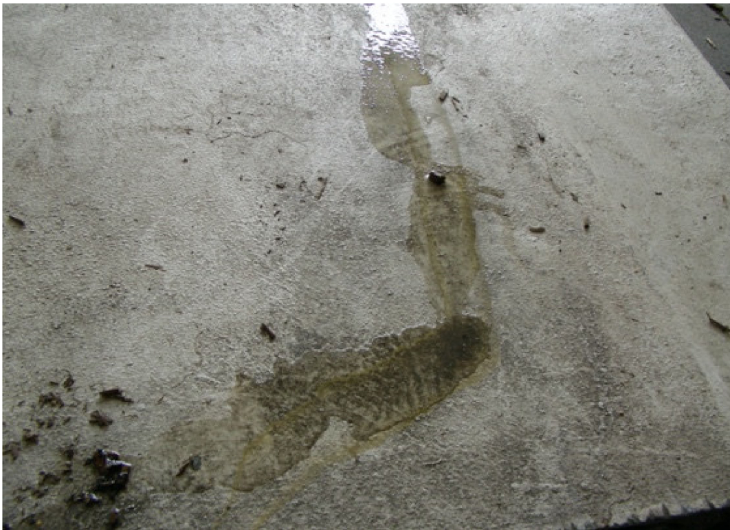
Figure 20. Blade lying horizontally working as a rain gutter, a yellow leach is visible (Photo by Piero Medici, 2011).
