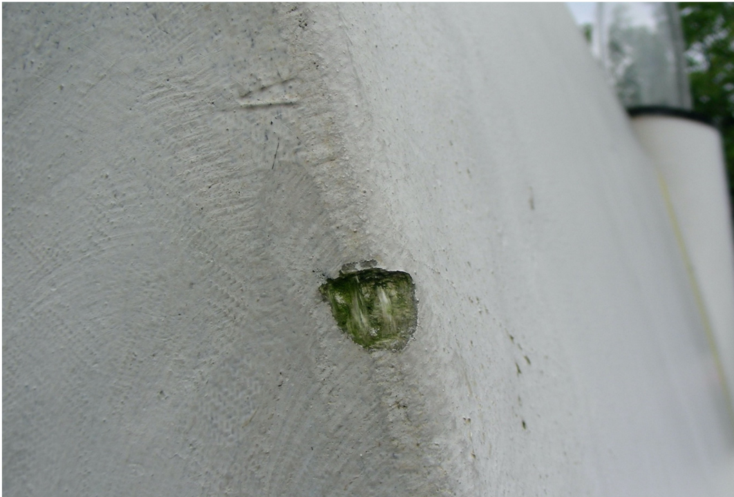
Figure 9. Damaged finish by Maropol, with glass fibres exposed, as a consequence of use damage (Photo by Piero Medici, 2011).
