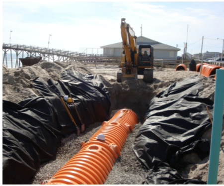
(a) Chambers of a dune infiltration system (Burchell et al., 2013).
