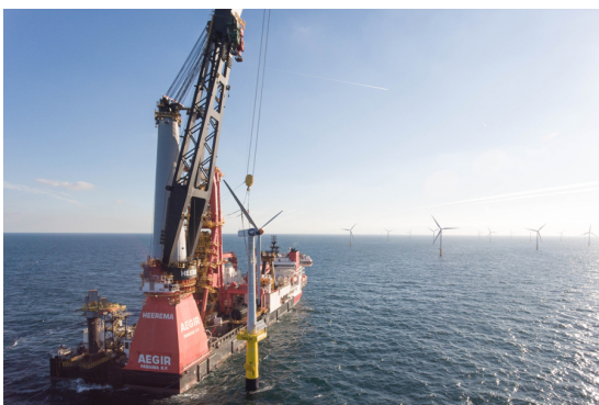
Figure 2.7: Installation of a WTG with a slip joint by a floating monohull.
