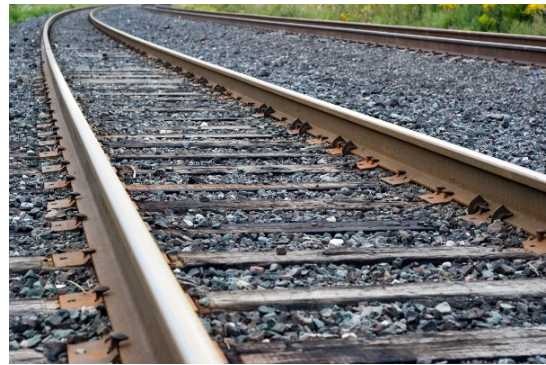
(b) Continuous Welded Rail track
