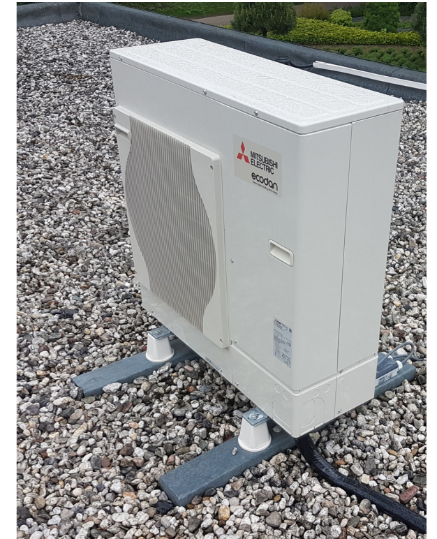
Figure 24. Images to give an impression of the heat pump installation set-up.
