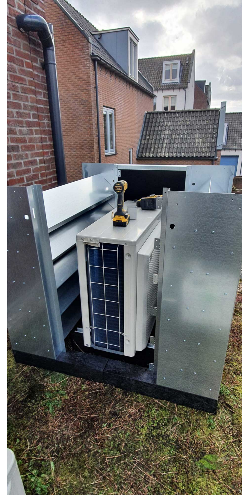
Figure 23. A heat pump installed on a green roof, in a casing to muffle the nuisance.
