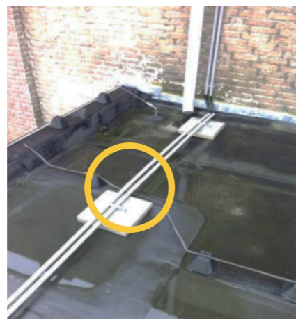
Figure 19. Faulty installed solar panels cables.
