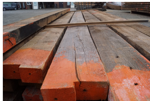
(b) Joint Notches at Item end and longitudinal Crack, Stack 4
