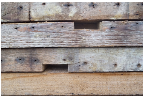
(a) Joint Notches and Nail Holes along the Item, Stack 4
