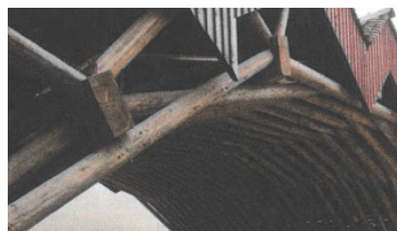
Figure 6.5: Joints of the Canopy in the Zhongshan Road Museum in Hangzhou, China, (Thönnissen, 2015)
