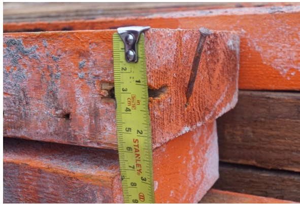
Figure 3.5: Nail remaining in RT Item, Stack 3
