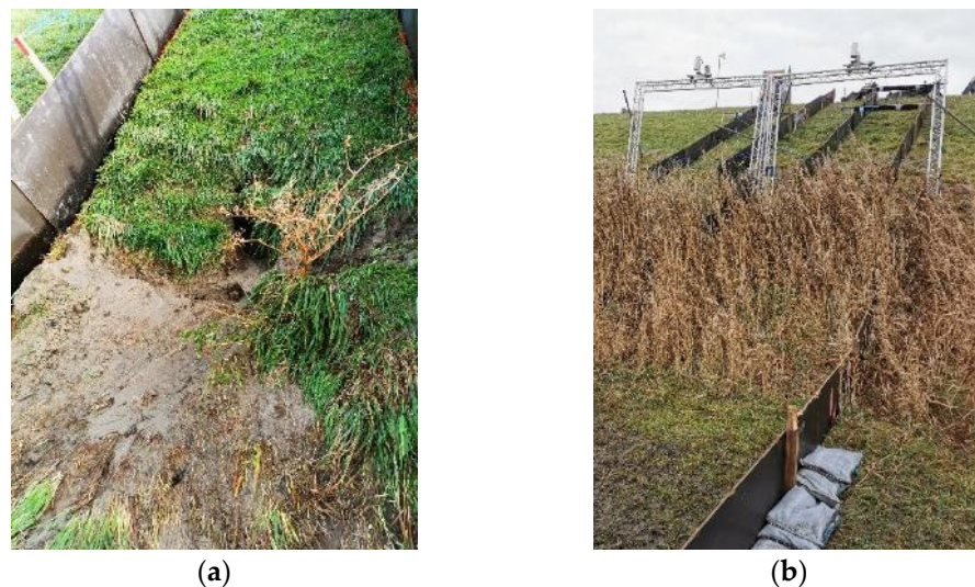
Figure 8. (a) Burrow entrance halfway the landside slope on a Dutch dike; (b) Sections with softened, saturated soil and reed overgrowth on a Dutch dike.
