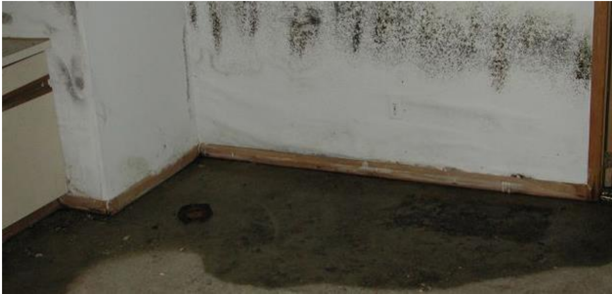
Figure 15: Small dewatering depth leading to rising damp that causes wet floors and walls (vochtproblemen-vochtbestrijding.nl)
