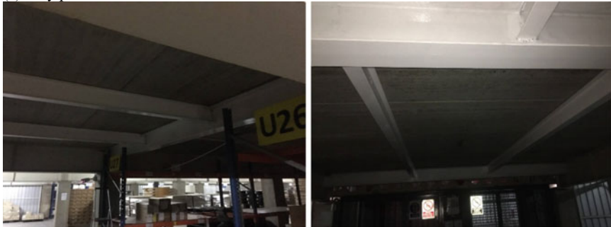
(b) Overview of the 1 st floor after installation of the steel beams
