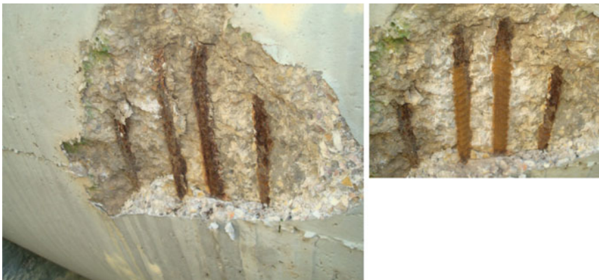
Fig. 5 Corrosion of the reinforcements in one of the pipes
