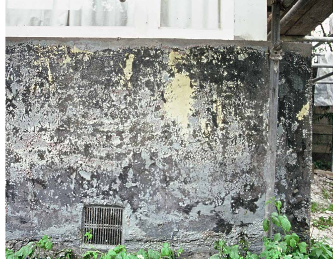
FIG. 2.9 Wall below the kitchen window in the east elevation; B. Mulder chose the dark grey of the top right corner for the new colour scheme
