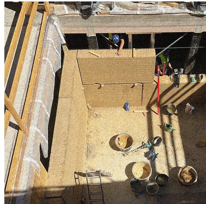
Figure 30 The final elements were stacked upon each other in a brick-like manner.
