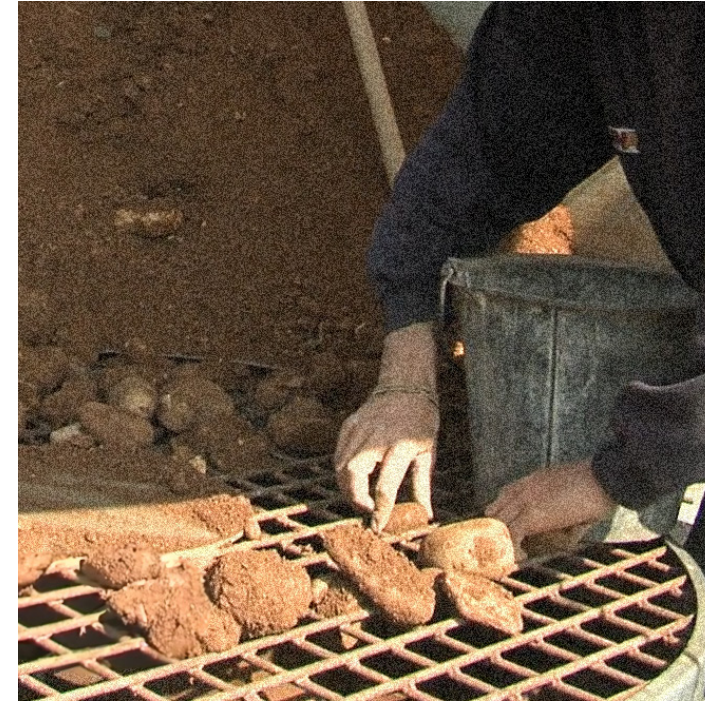
Figure 34 The sieve sorts out larger stones that are unsuitable for the mixture.
