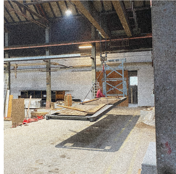
Figure 11 Prefabricated elements are transported with inloaders. The inloader palette is lifted with a crane on tracks.
