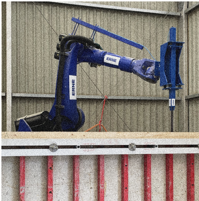
Figure 28 The robot reaches over and inside the formwork to compact the layers.
