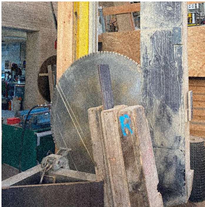
Figure 19 In the end, the 40m long prefabricated wall gets cut up into the required lengths.
