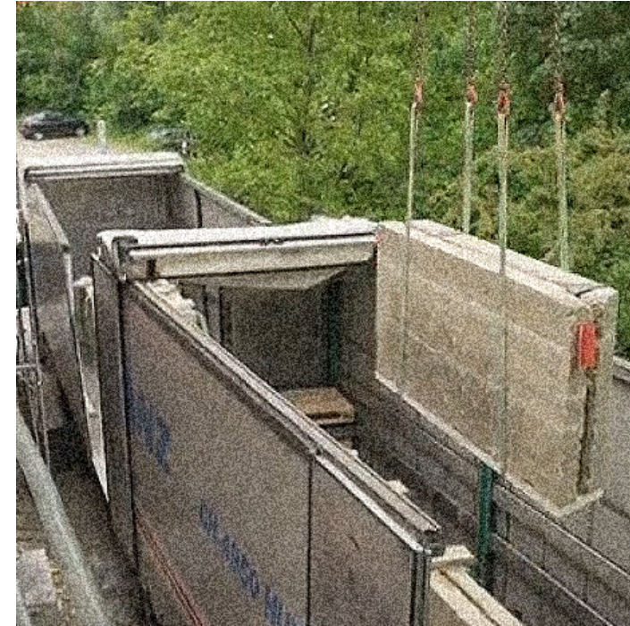
Figure 20 The finished elements are transported via truck and lifted to the final position on the construction site.
