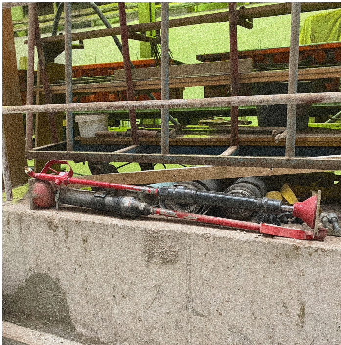
Figure 10 Two manual pneumatic tampers are used to further compress each rammed earth layer.
