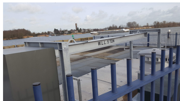
(b) The removable lifting frame above culvert number 3.
