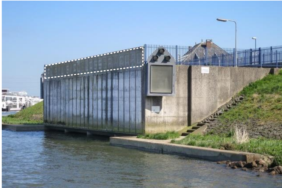
Figure 11.4: Letters on the outer wall of the Elshoutsluice saying Spuisluis Alblasserwaard (translated: discharge sluice Alblasserwaard). The outline of the letters is marked. Source: https://beeldbank.cultureelerfgoed.nl/ .
