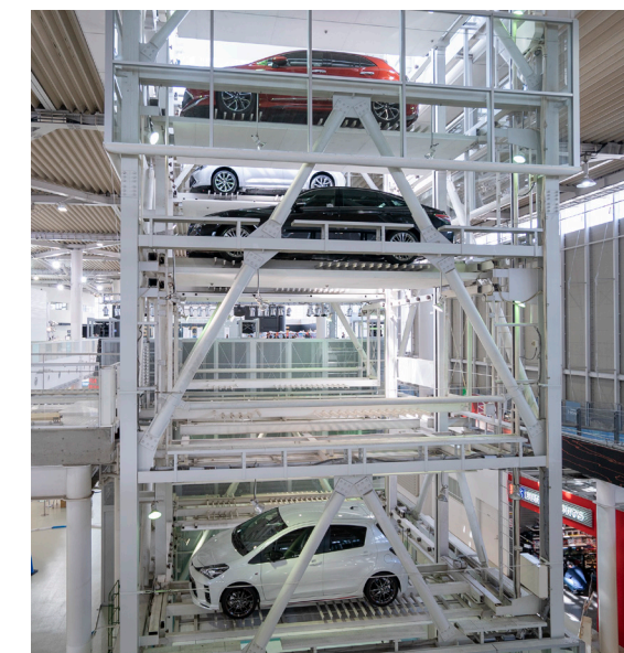
Figure 81.2 - Will mechanical parking lots cease to exist when AV valet parking will be widely adopted?
