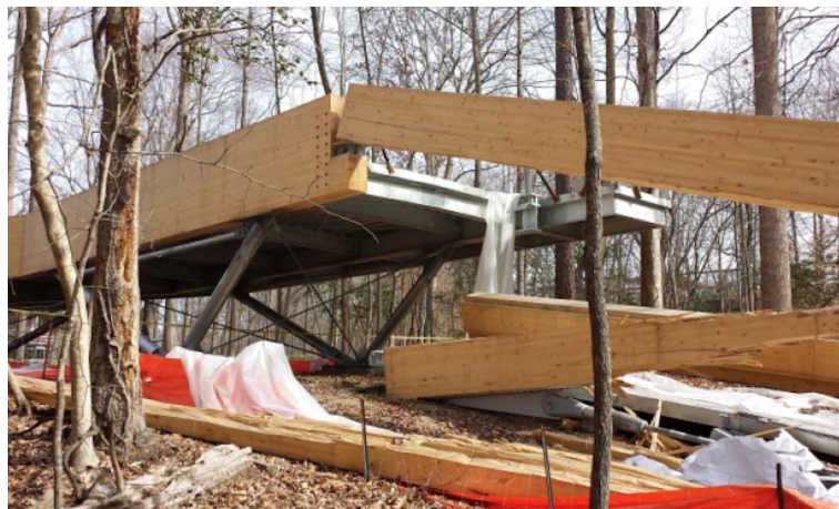
Figure 1.1: Wake Tech Community College timber bridge collapse. From (Van Voorhis, 2016).
