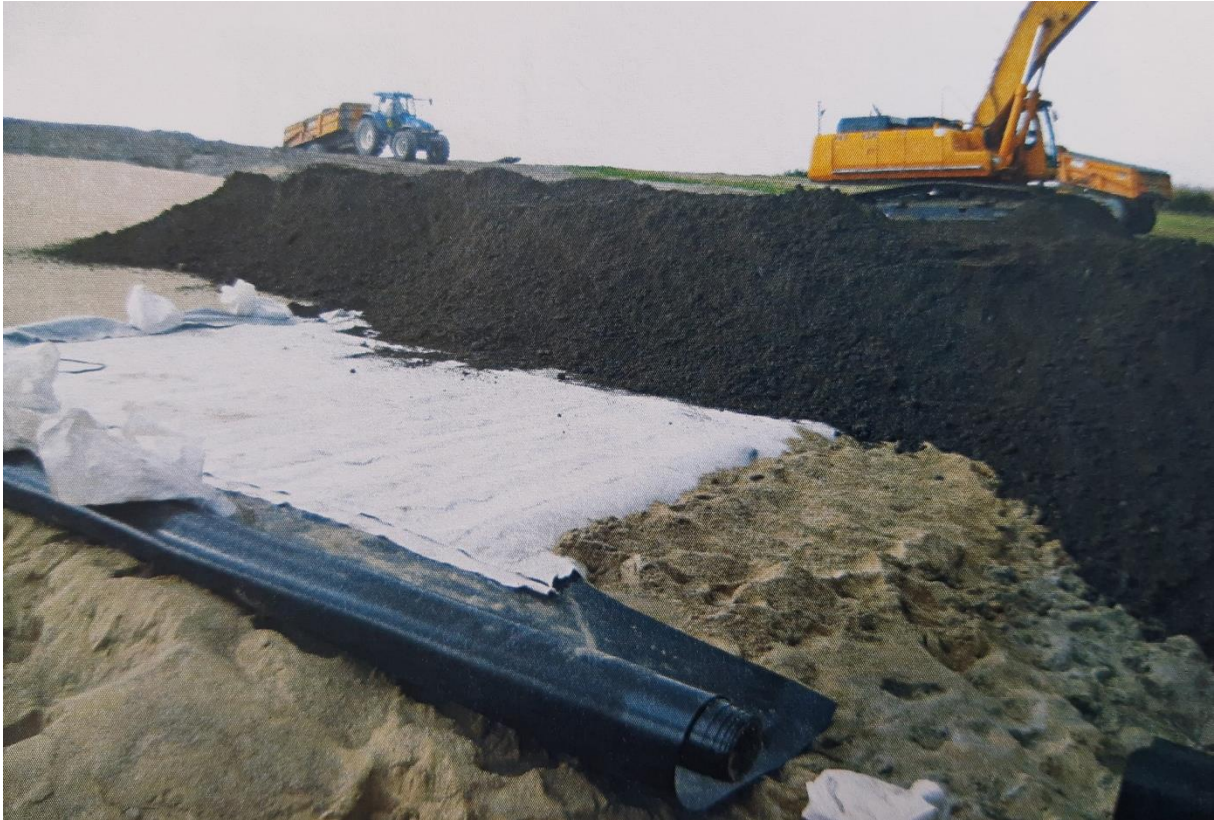
Figure 34: Construction of MOL. The white mat is a drainage mat above the drain for the CL, to prevent additional precipitation to be collected.
