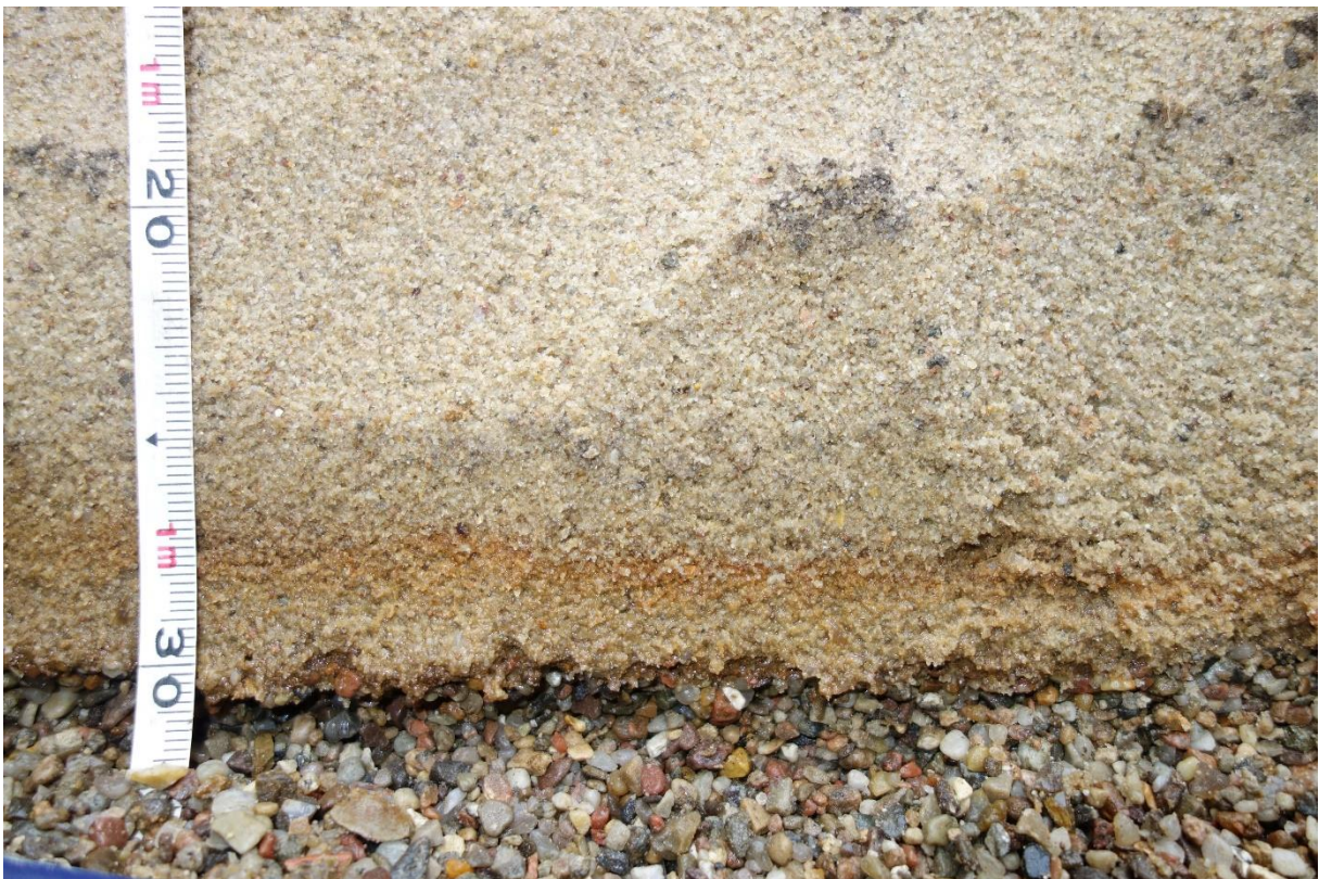
Figure 52: Excavation November 2017: formation of most likely iron precipitates at the bottom of the CL (Verseveld, 2018). As there were also iron precipitates in the outflow of the CL and CB, it is most likely that most of the CL flow happened at the bottom 3-4 cm.
