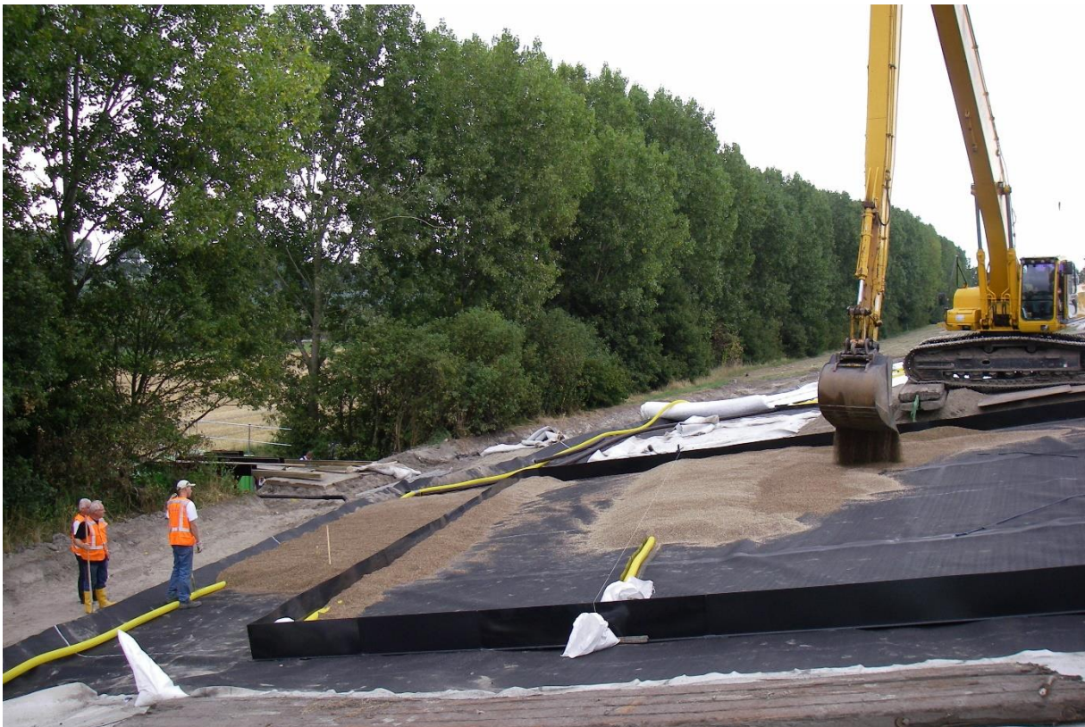
Figure 31: Construction of the capillary block, which drains through the most upslope drain. The capillary layers drains at the bottom drain.
