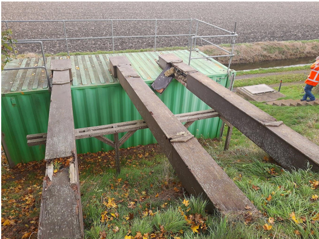
Figure 41: The insulated drainage pipes of the capillary layer and block (left two pipes) leading to the measurement container.
