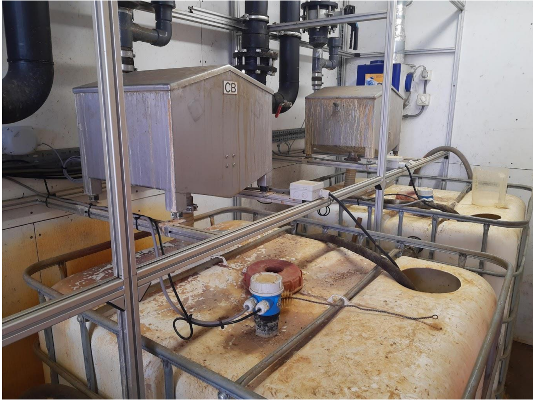
Figure 42: Inside the measurement container the tipping buckets and the IBC water storage tanks.
