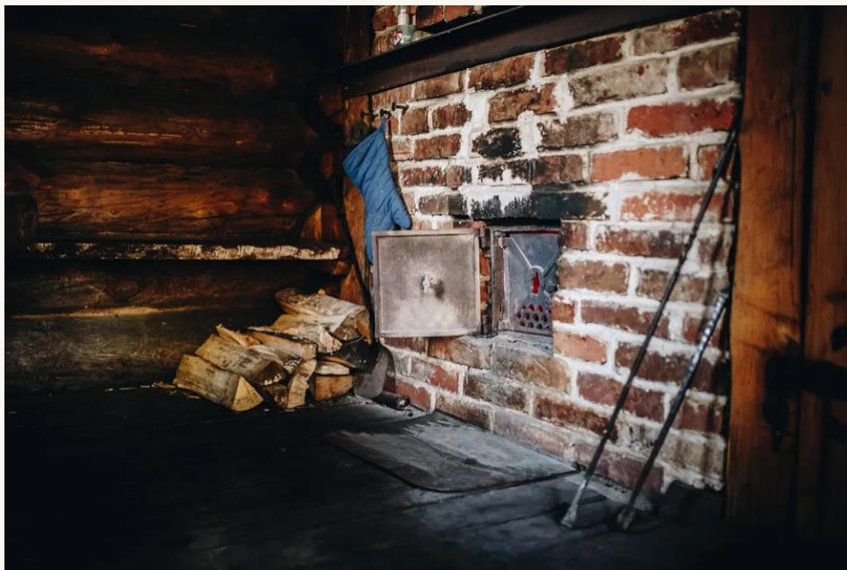
Figuur 1. Wood-fired sauna oven.
