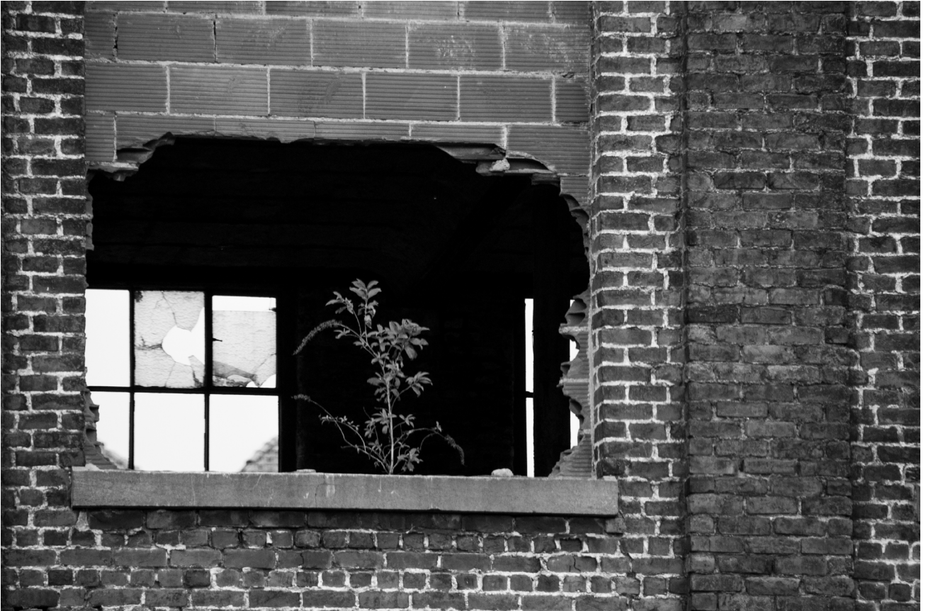
Ruins of the former textile factory Desurmont et Fils by author. 2017. Tourcoing, France
