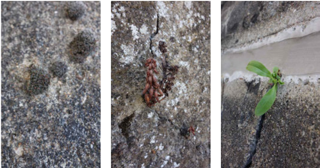
FIG. 5.13 The existing plants found on the roof Tiny plants inhabit the shade or the crevices of the concrete surface, resisting the dry micro-climate on the roof.
