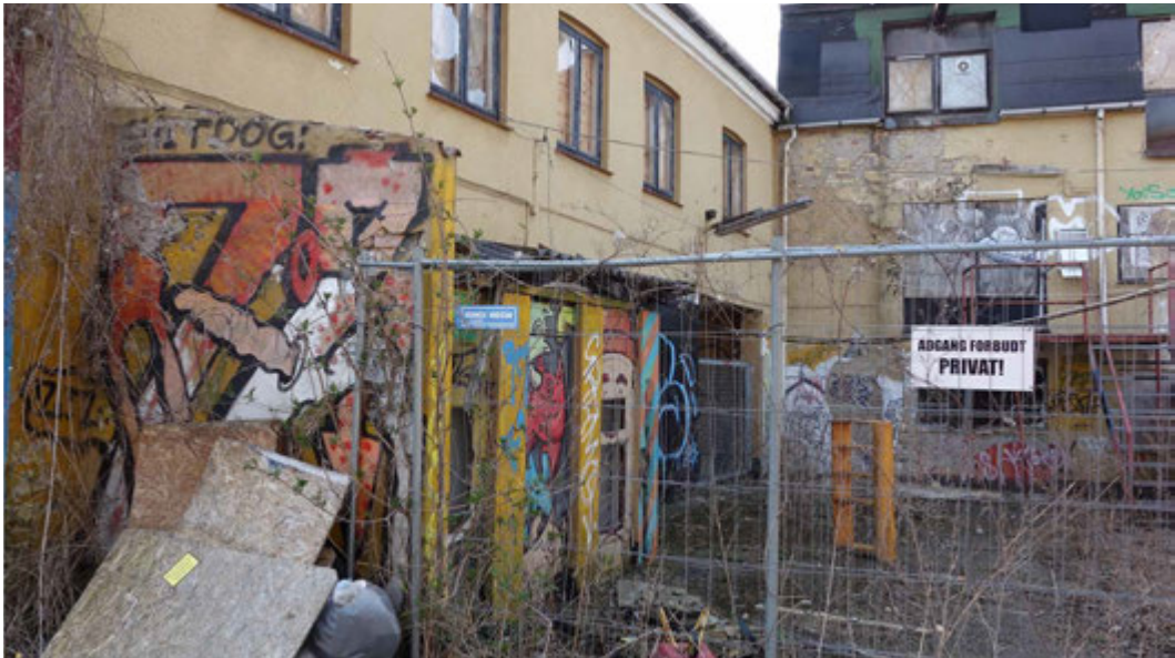
FIG. 4.24 / B The material world of the site during site visit in April 2017 The backyard is rather dilapidated, filled with deteriorated objects, materials, and graffiti.
