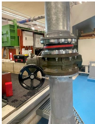
Figure 4-25: Valve of inflow pipe
