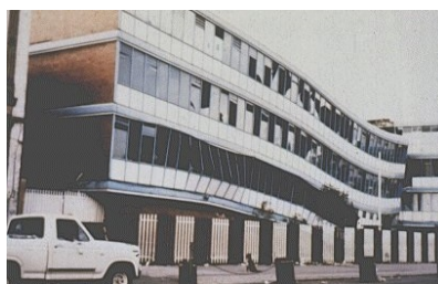
Figure 2.7.: A building in Mexico City which failed due to torsion (Earthquake Engineering ANNEXES, 2007).
