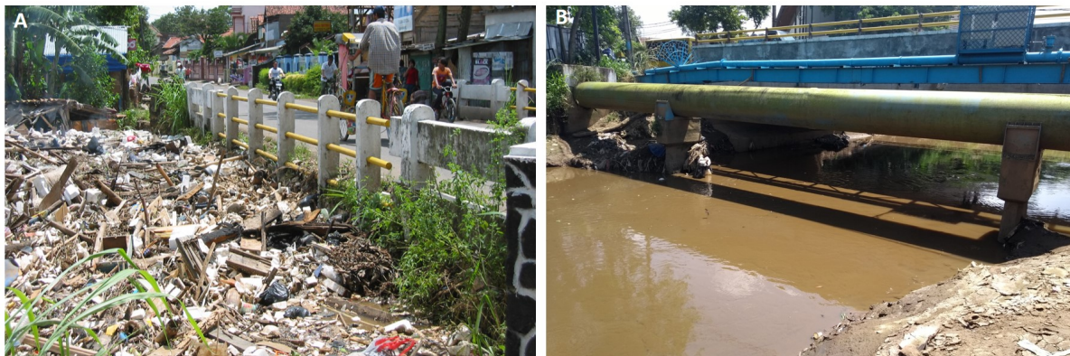
Figure 1.3: (A) Debris bridge blockage in Cikapundung River in January 2010 (Ministry of Public Works and Housing, 2010), compared to (B) the regular flow condition at the same bridge in May 2018.
