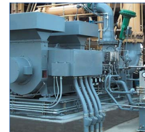
Rotoflow recently modified an axial turbine at a geothermal facility in the western US to a radial turboexpander.
