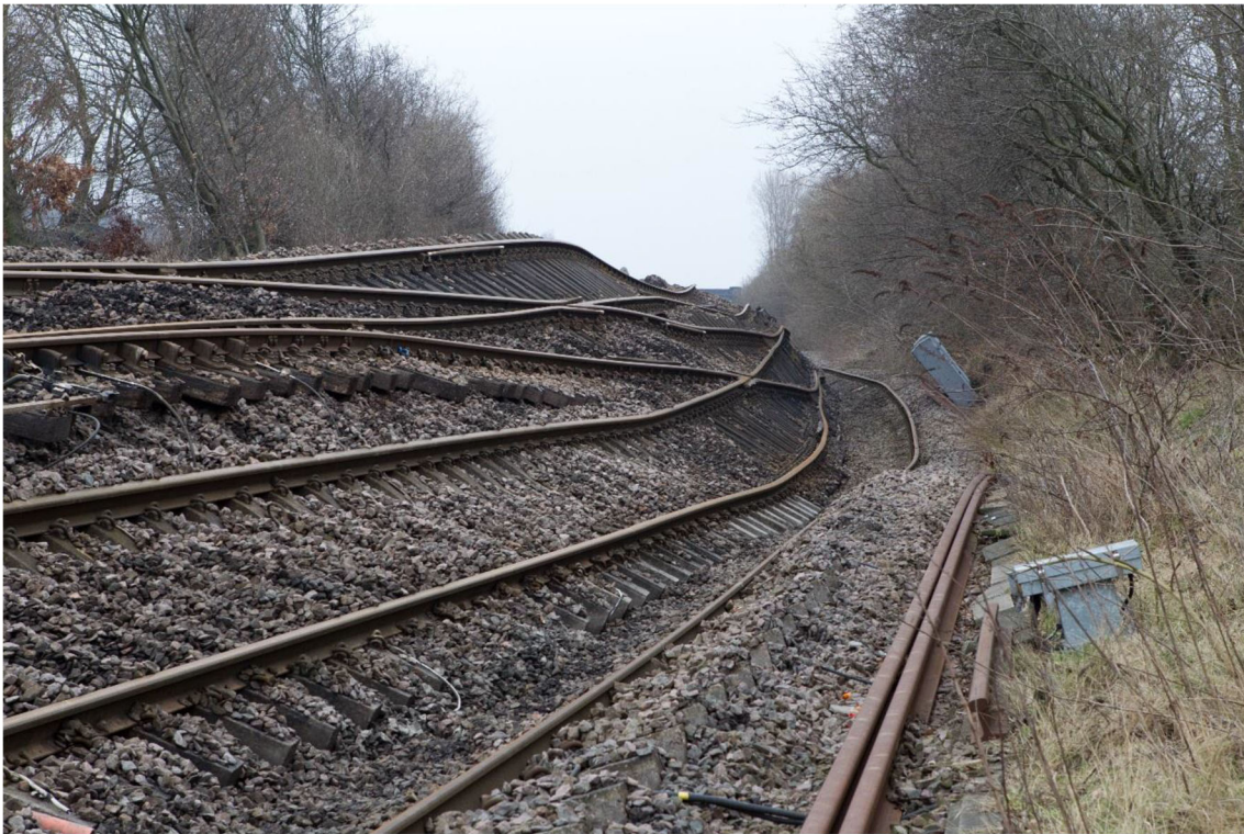
FIGURE 3 Landslip near Hatfield Colliery, UK, February 2013. Image © Network Rail
