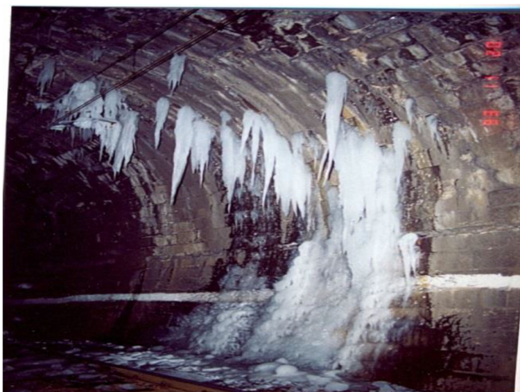
FIGURE 6 Ice formation in rail tunnel, Slovenia; after Gavin (2016)
