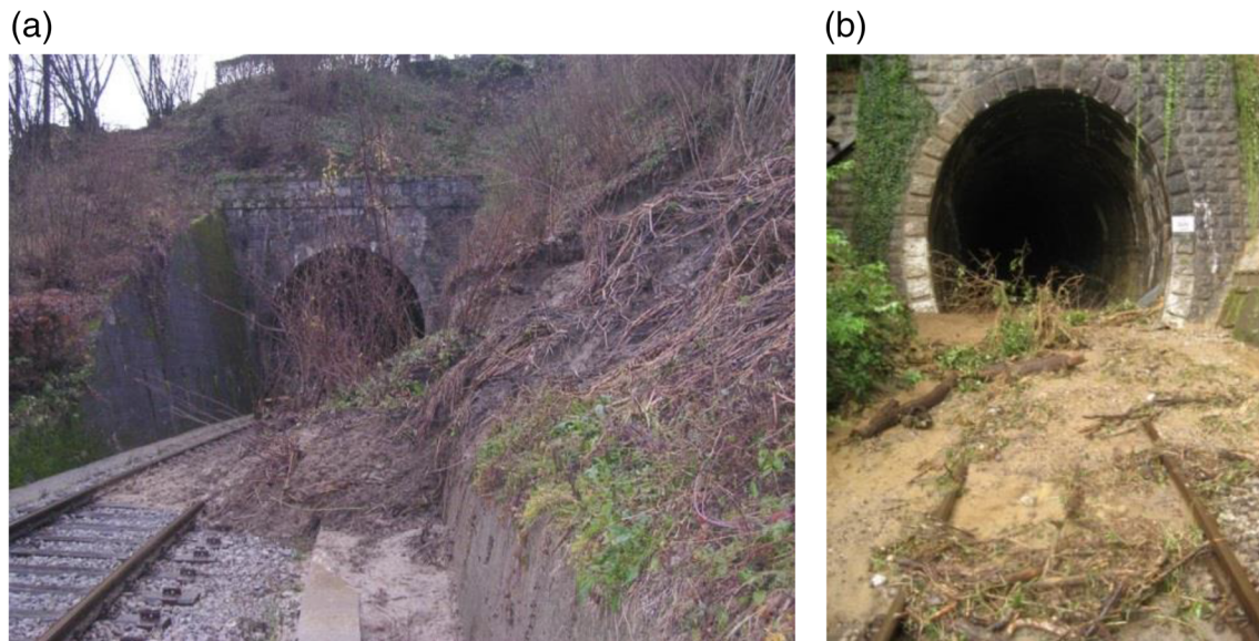
FIGURE 2 (a) Shallow landslide on the Ljubljana-Kamnik line, Slovenia. (b) Failure at the Zaluka Tunnel, Croatia, on the Karlovac-Kamanje line. After Gavin (2016)
