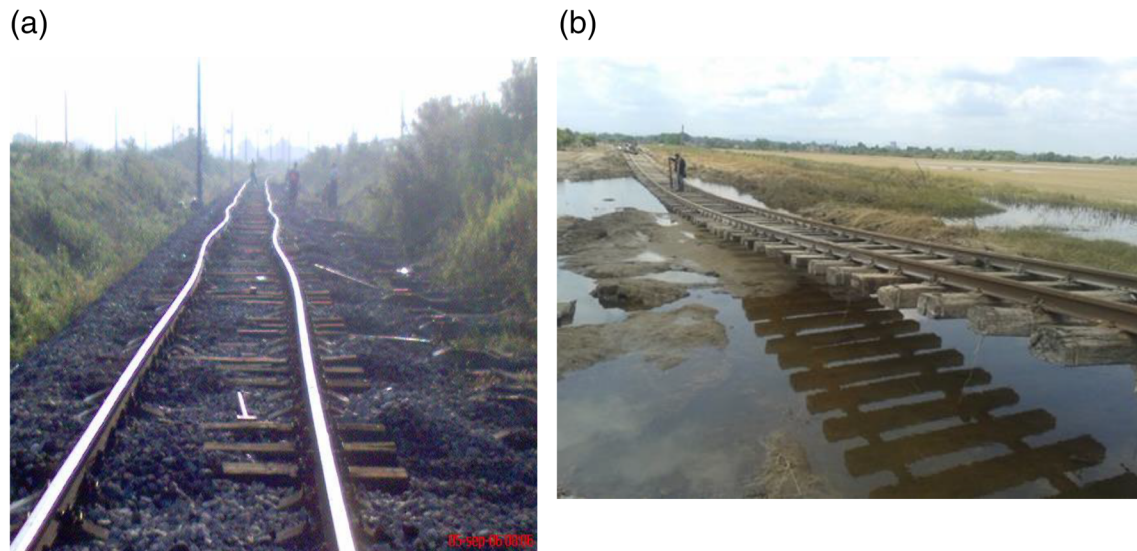
FIGURE 7 (a) Lateral buckling of the track due to high temperatures, Slovenia. (b) Embankment scour at Krušljevac, Podrute on the Zaprešič-Čakovec line (Gavin, 2016)
