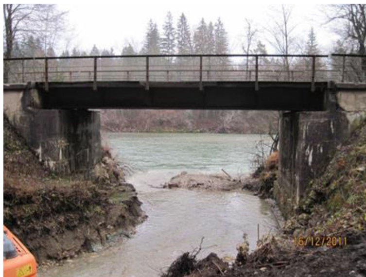
FIGURE 8 Scour of foundation at Plaznica bridge on the line between Ljubljana and Jesenice (Gavin, 2016)
