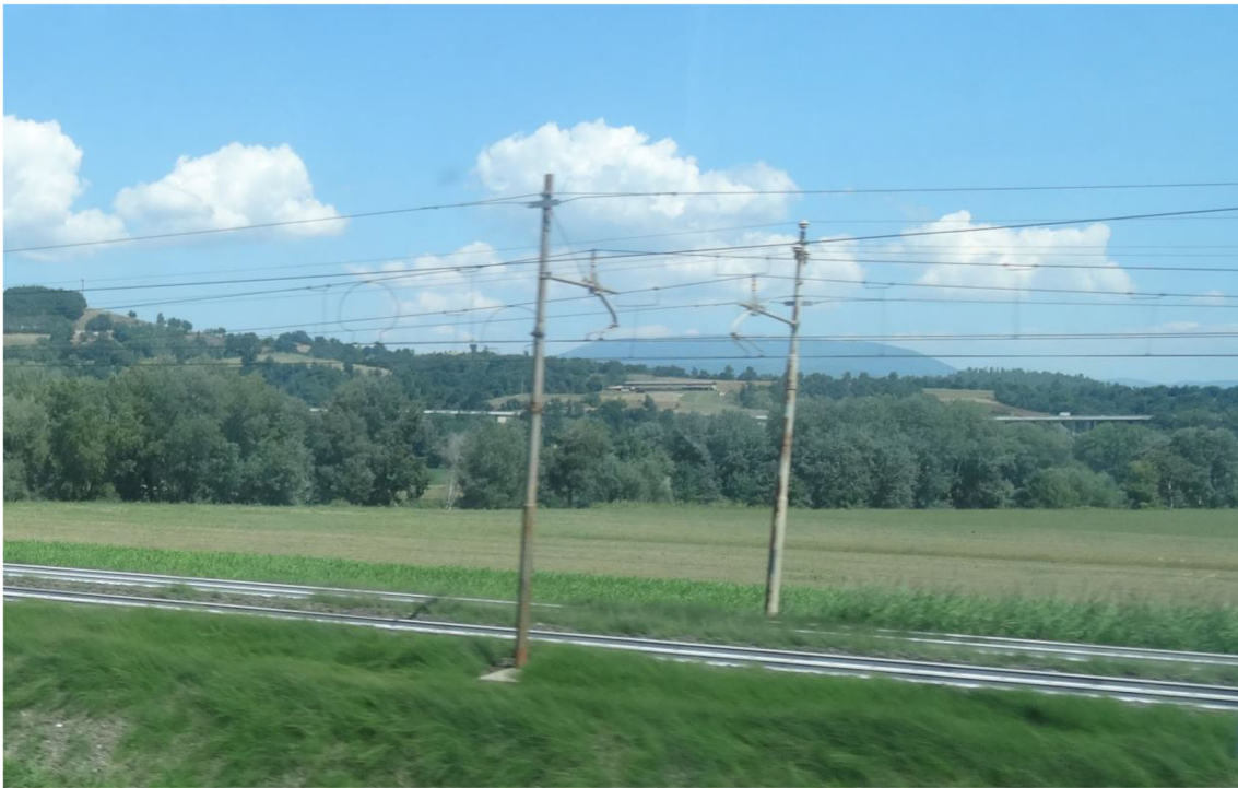
FIGURE 12 Italian railway, with rails painted white to reduce buckling risk. Image courtesy of Peter van der Linden—used with permission
