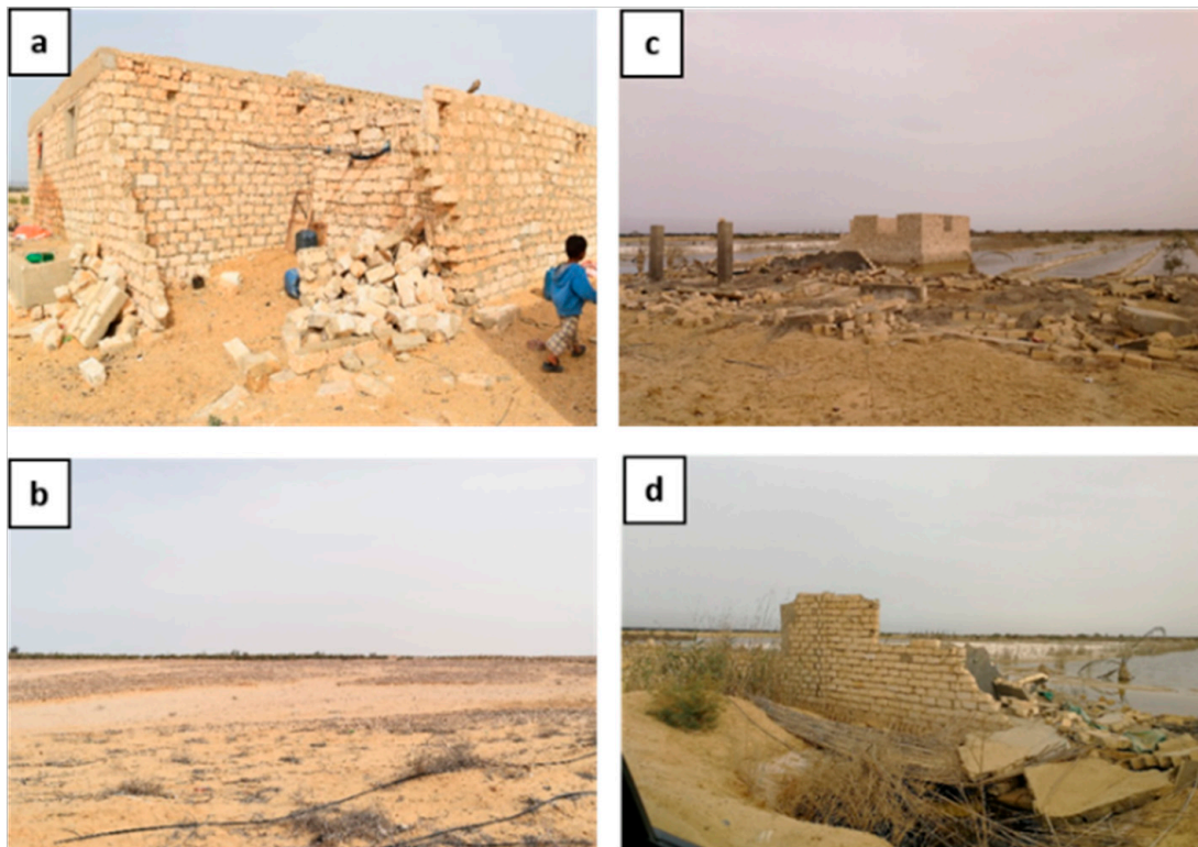
Figure 3. Consequences of a flash flood at Afouna Village: (a) damage to property, (b) one of the main flood stream paths in the village, (c) destruction of agricultural land, (d) wall collapsed in the main road.
