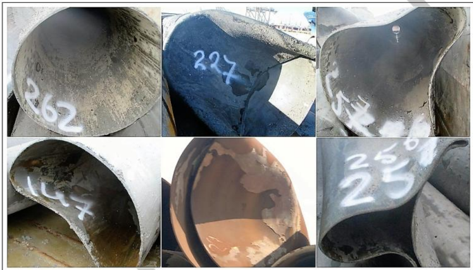
Fig. 2 Various types of damages to the tubular piles [10]
