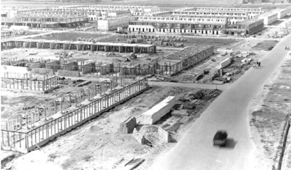
Figure 4. Nemavo-Airey system. Construction of the residential neighbourhood of Jeruzalem in Amsterdam (1950). Source: Stadsarchief Amsterdam.
