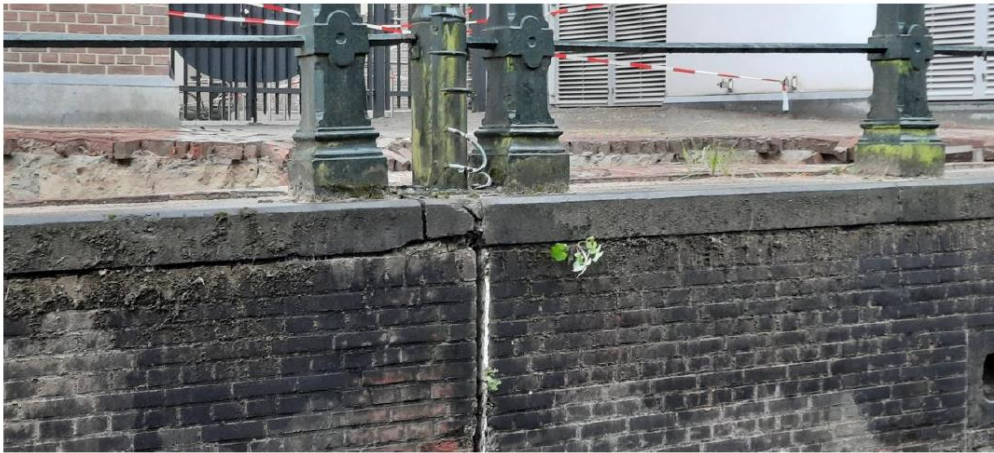
Figure 2.4: a dilatation joint in the Grimburgwal from the research of Korff et al. (2021).
