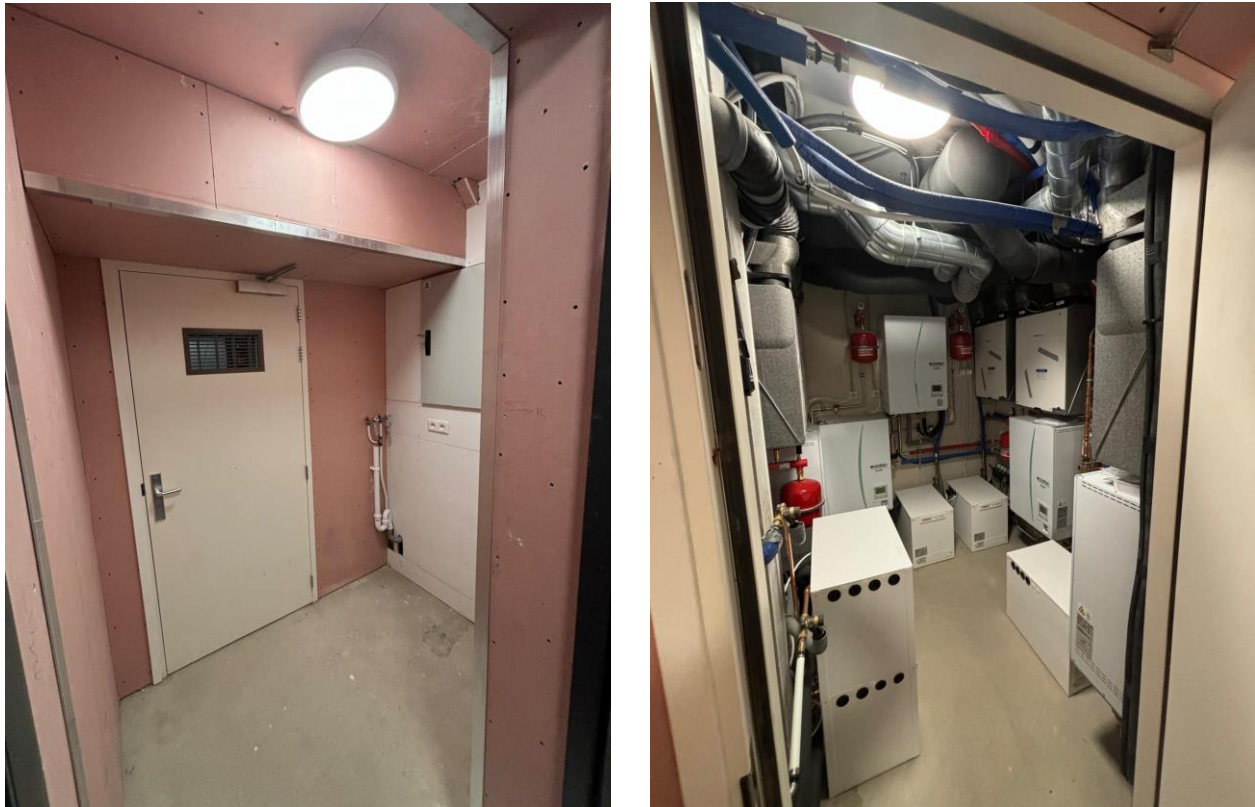
Figure 5.34: Centralized technical room (own photo, 2024)
