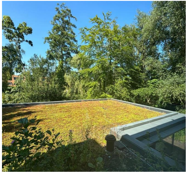
Figure 5.26: Green roof (own photo, 2024)
