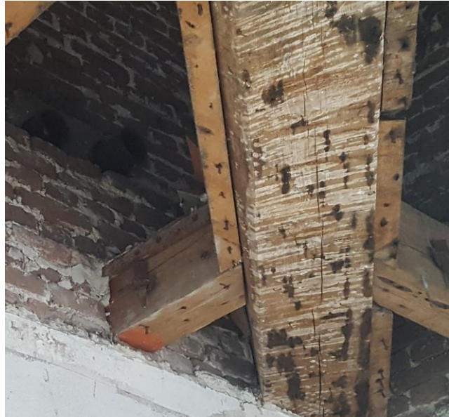
Figure 5.10: Rotten wooden beams (Res & Smit BV, 2016)
