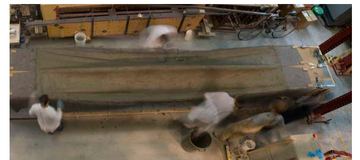
Figure 30. Prototype for a "flayed beam" being cast on a hung mold (Source: Mark West / C.A.S.T.)
