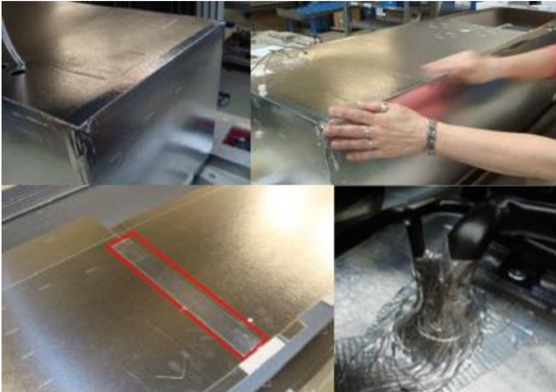
Figure 41: all the location where the expensive fire retardant duct tape is used (yes, this is the only the wrapper)
