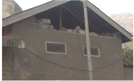
Figure 1.6: Typical overturning of the top of the wall (source: Javed et al., 2006)
