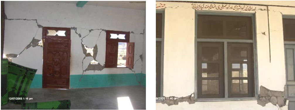
Figure 14: Diagonal cracks and rocking in masonry piers, left and right respectively (source: Javed et al., 2006)
