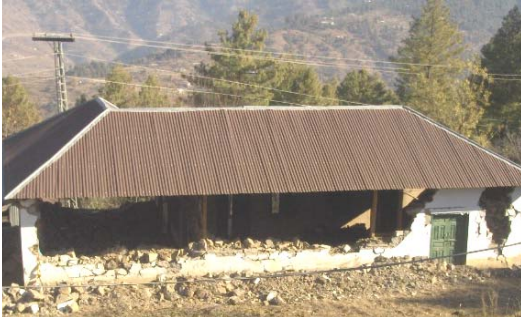
Figure 1.5: Total collapse of an out-of-plane loaded wall (source: Javed et al., 2006)
