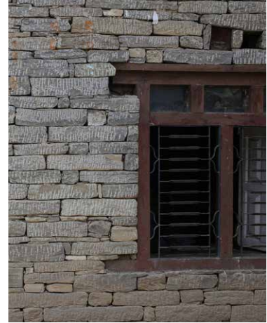
Figure 6.14: Typical Nepali window: timber frame connected to the masonry by interlock (source: own photo).
