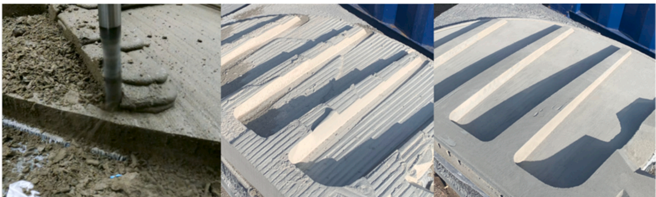
Fig. 25. Milling a 3DCP panel to create accurate and precise feature details while the printed material is in its green state (left); and the resulting impact on the aesthetics of the hardened component, partially milled (centre), and fully milled (right). (For interpretation of the references to colour in this figure legend, the reader is referred to the web version of this article.)
