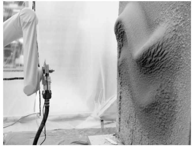
Fig. 6. Robotic Plaster Spraying (RPS) introduces a gravity-resisting, vertical thin-layer spray-based printing technique (ETH Zurich, 2021) [30].
