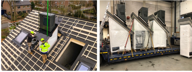
Figure 10.11 Preassembled building services unit placement on the roof. Factory Zero, the Netherlands, energy modules.
