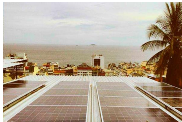
Figure 14. “Escolinha Tia Percília” PV power plant (2019). Source: Revolusolar .
