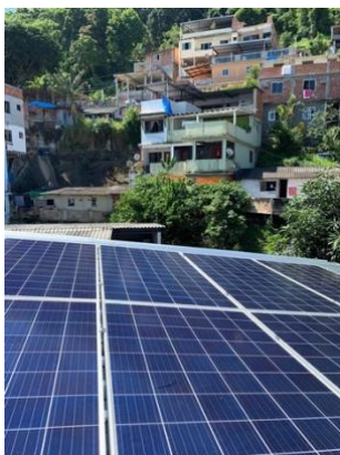
Figure 12. “Babilônia Rio Hostel” PV power plant (2016). Source: Revolusolar .
