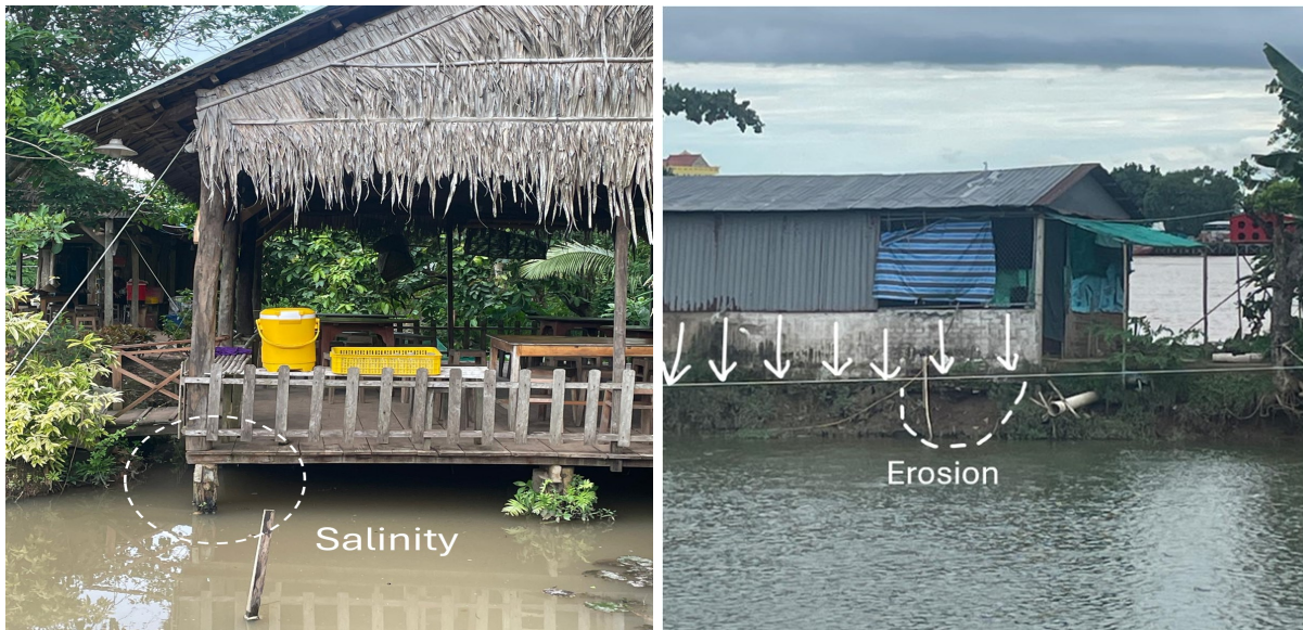
(a) Salt affecting the foundation pile
