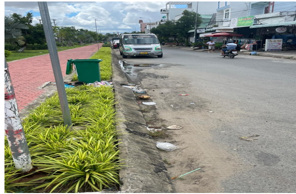
(b) Waste in the sewage pit
