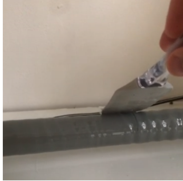
(b) Spreading the silicone evenly across the pipe with a silicone spatula to ensure uniform thickness.
