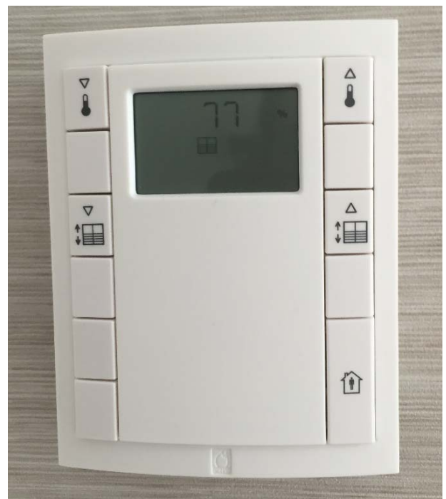
Figure 3. Thermostat and control blinds.
