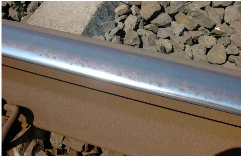
Fig. 2. High rail running surface at site A – situation prior to rail replacement (traffic direction to the right; depicted rail length about 0.36 m).
